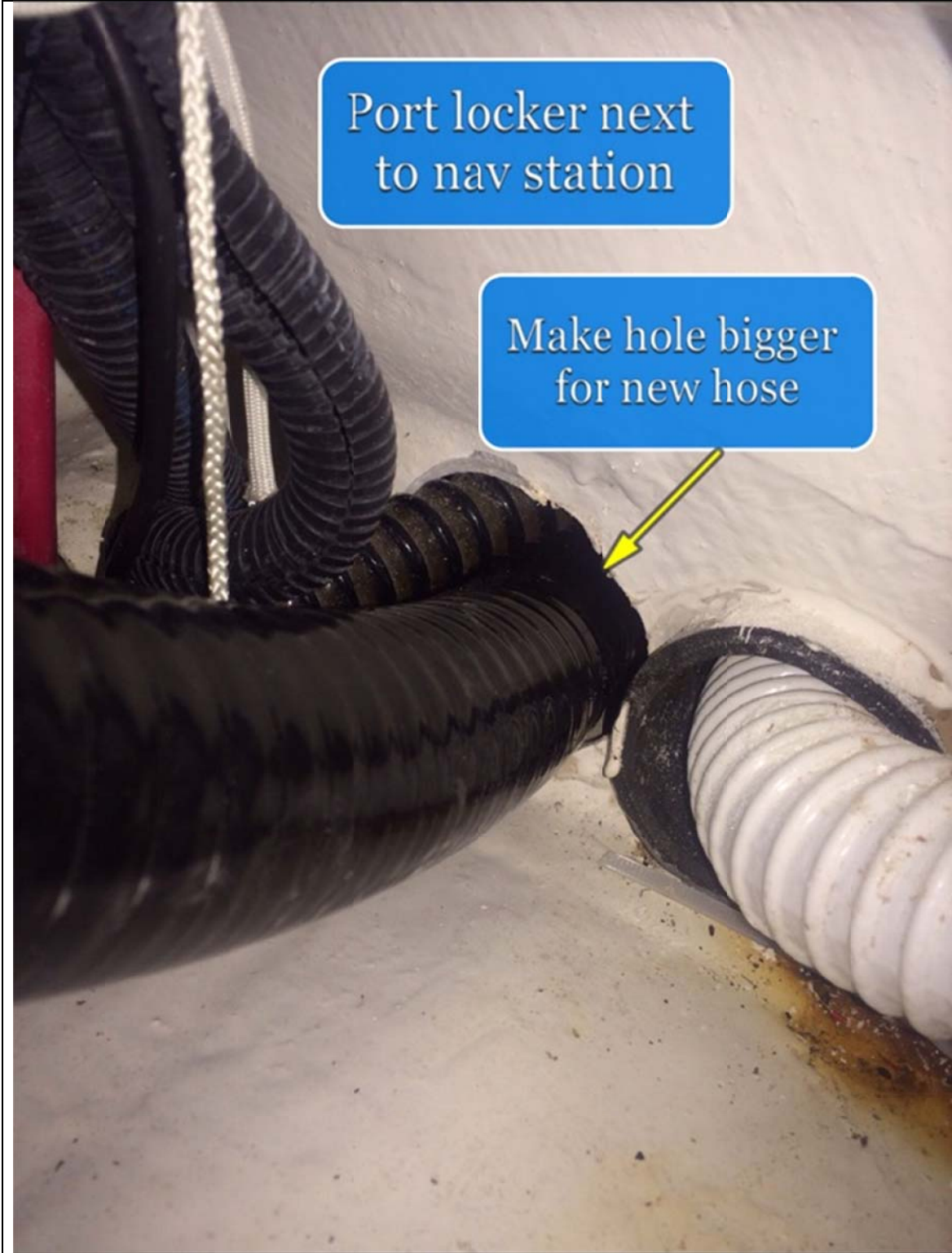
The new 1.5 inch hose needs to go into the bilge pump locker next to the have station. The hole need to be opened up and we can just get the hose into the bilge.
