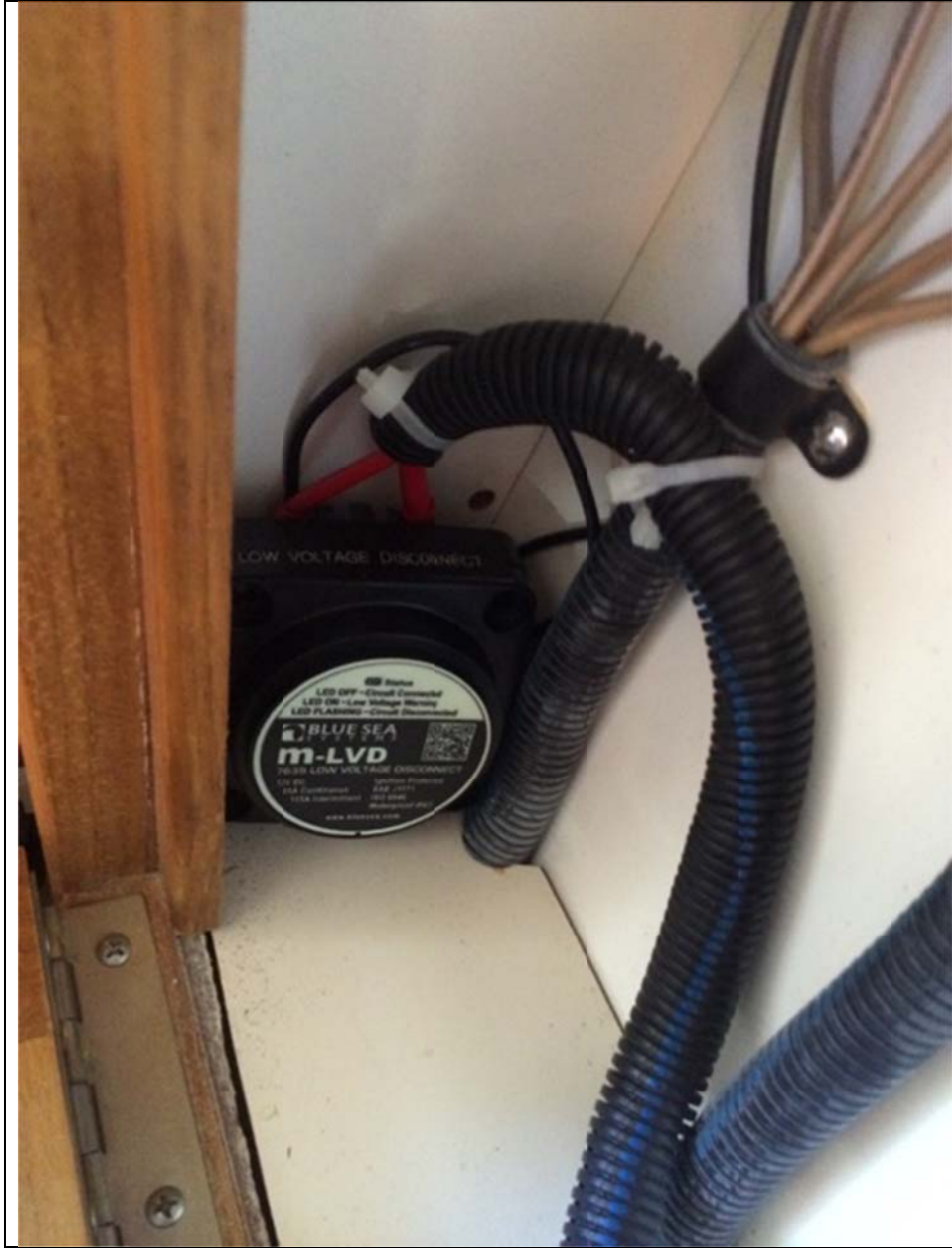
It just fits in the corner of the panel. Then tie wrap it down.
